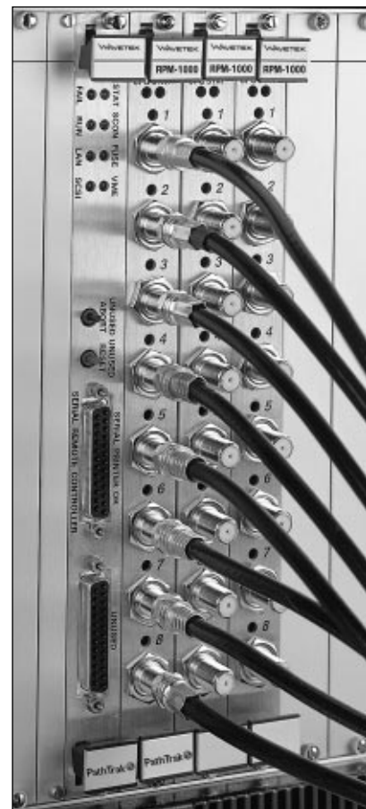
Close-up of modules on back of the HCU1500.
