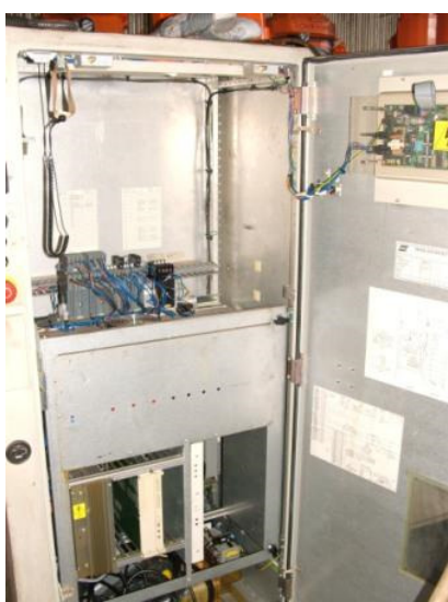
Inside the S3 controller
